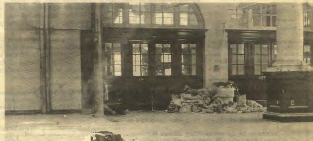
The main floor—the first sight to greet visitors are the piles of old plaster awaiting a decision on the future of the Duckworth Street building.
